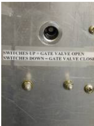
Figure 3 – Gate valve open/close switches
